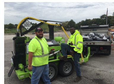
(Left) Daniel Vandebos and (Right) Ron Harper prepare to crack seal Roeland Park Streets. An unwritten value in Roeland Park PW is to have fun.
